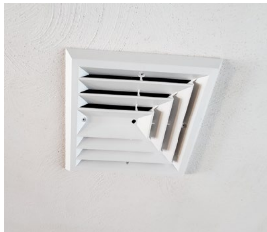
Ducted ASHP heating and cooling vent
