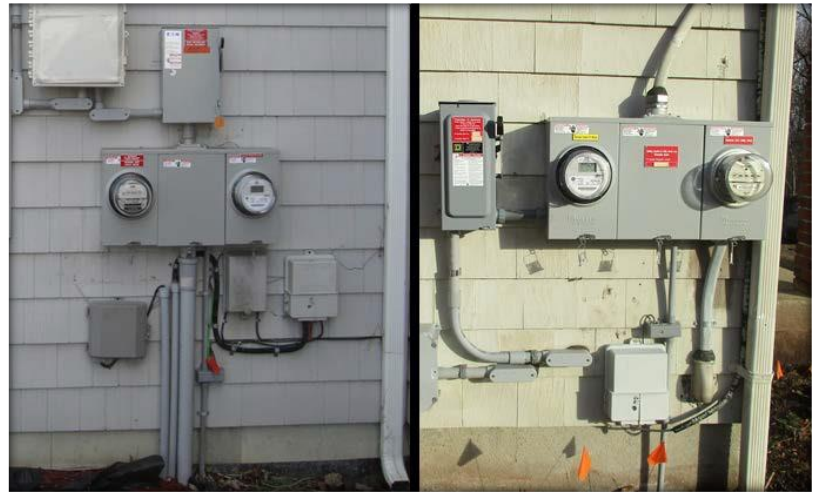
Figure 3. New Multi-Gang Meter Enclosures in Existing Underground (left) and Overhead (right) Electrical Services
