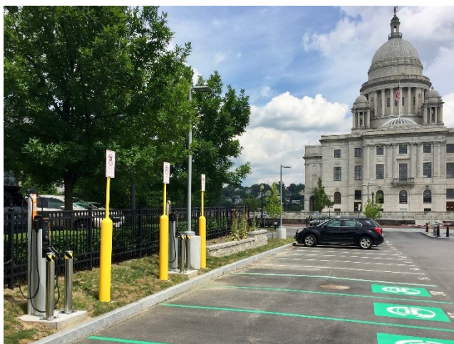
Figure 3. EV Chargers in front of Capital Building
