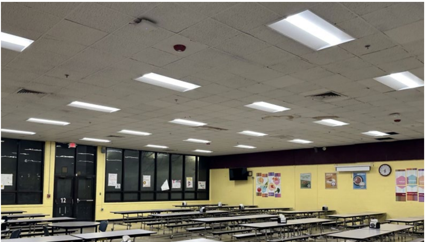
LED lighting was installed at five schools in Pawtucket, RI.
