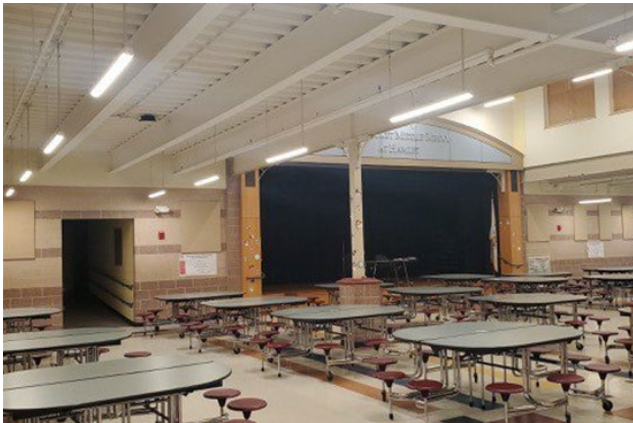
Cafeteria at Pothier Elementary School with LED lighting
