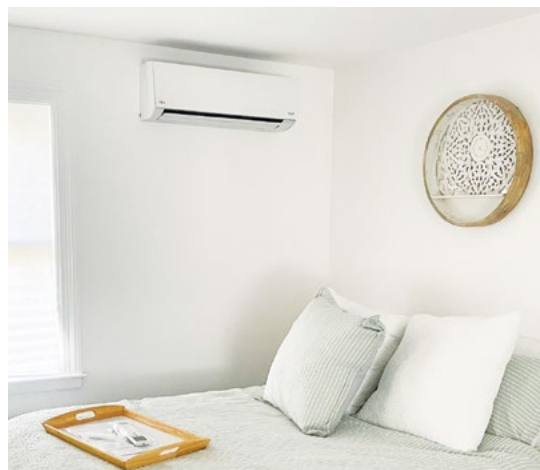
Ductless ASHP indoor wall unit
