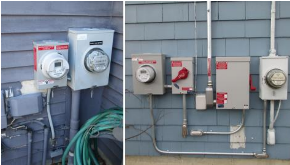
Figure 6. Connections Made In Existing Meter Enclosures on (Left) Underground Service Laterals, and (Right) Overhead Service Drops
