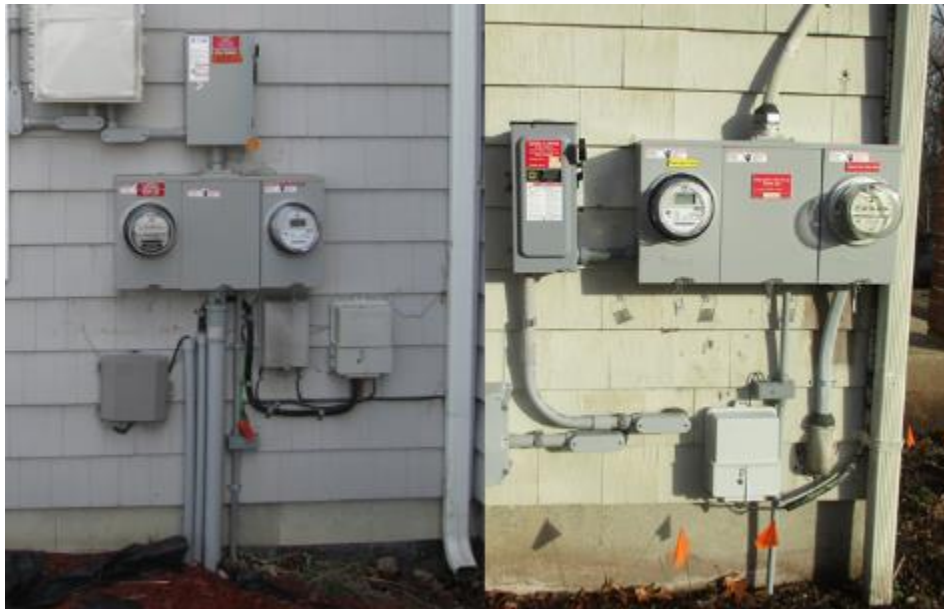
Figure 4. Example of New Multi-Gang Meter Enclosures Installed in (Left) Underground Service Laterals and (Right) Overhead Service Drops
